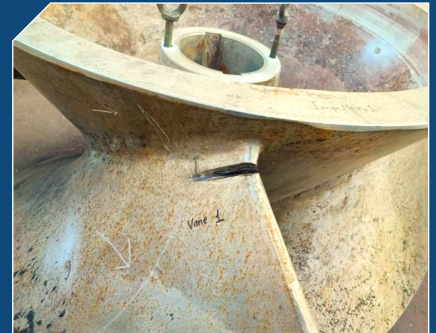
Crack on Impeller
